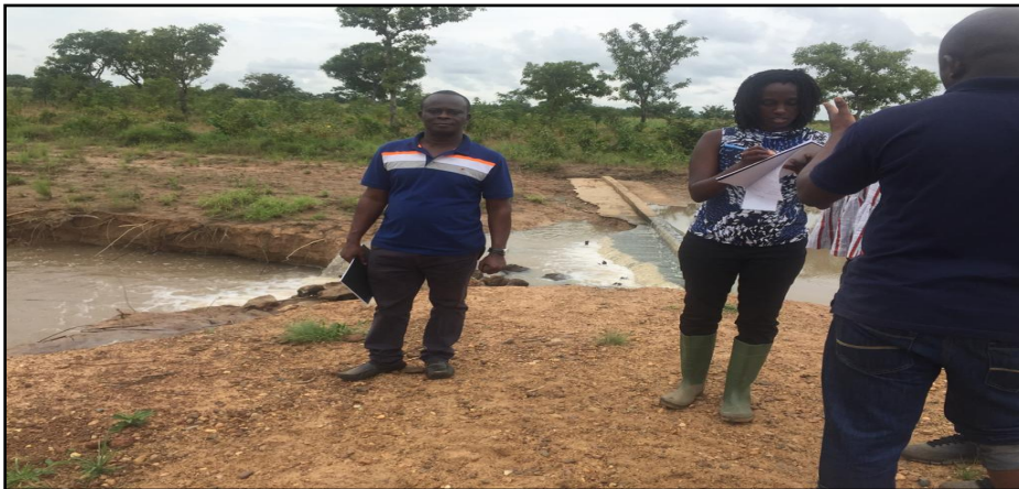
Figure 8: Broken spillway of a dam in Kulikpegu- Mion District
