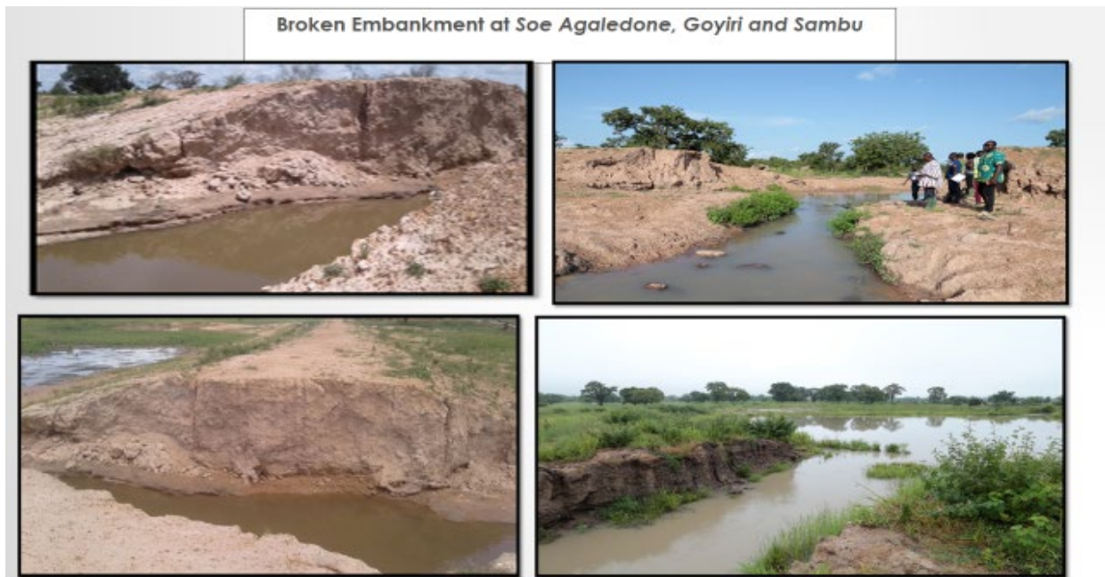
Figure 7 : Broken Embankment at Soe Agaledone, Goyiri and Sambu
